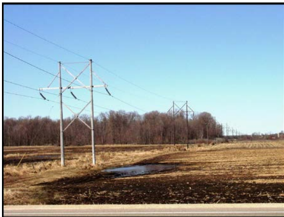
Figure 1 Typical Two-Pole, H-frame Structure
